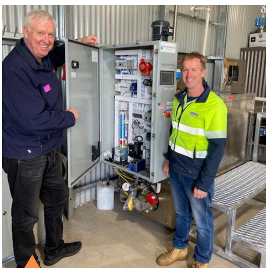
THE INSTALL: VETERINARIAN ALKALINE HYDROLYSIS MACHINE (PET-550) WITH CUSTOM 3 PHASE TRANSFORMER
