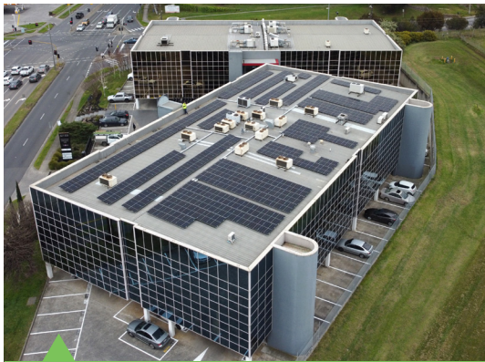
THE INSTALL: 100KW SOLAR PV SYSTEM
