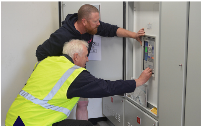
BEFORE & AFTER: SEAN MOORE, OWNER RED'S ELECTRICAL & HANK TERPSTRA, MIDDY'S INDUSTRIAL BUSINESS DEVELOPMENT MANAGER
