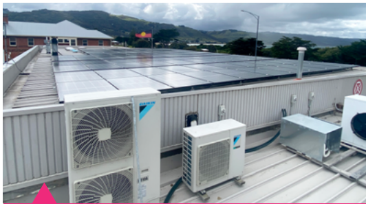
THE INSTALL: 36KW ROOF MOUNT SOLAR SYSTEM
